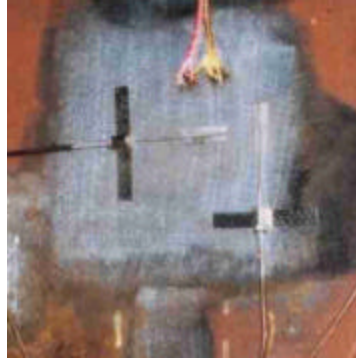
Hoop and Axial HTSG with separated junction TC on Coke Drum
