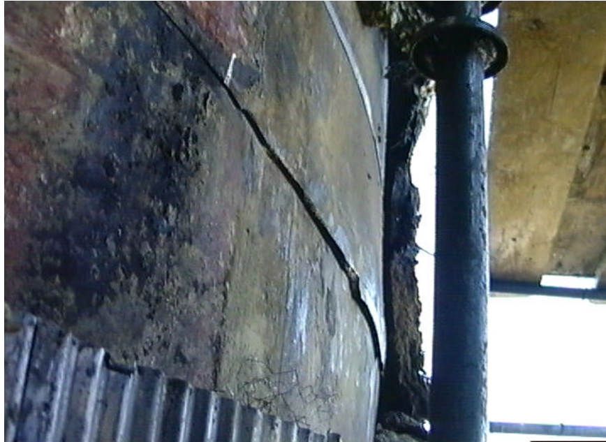
Extensive through-wall OD cracking at recently repaired circ weld, started from inside.
